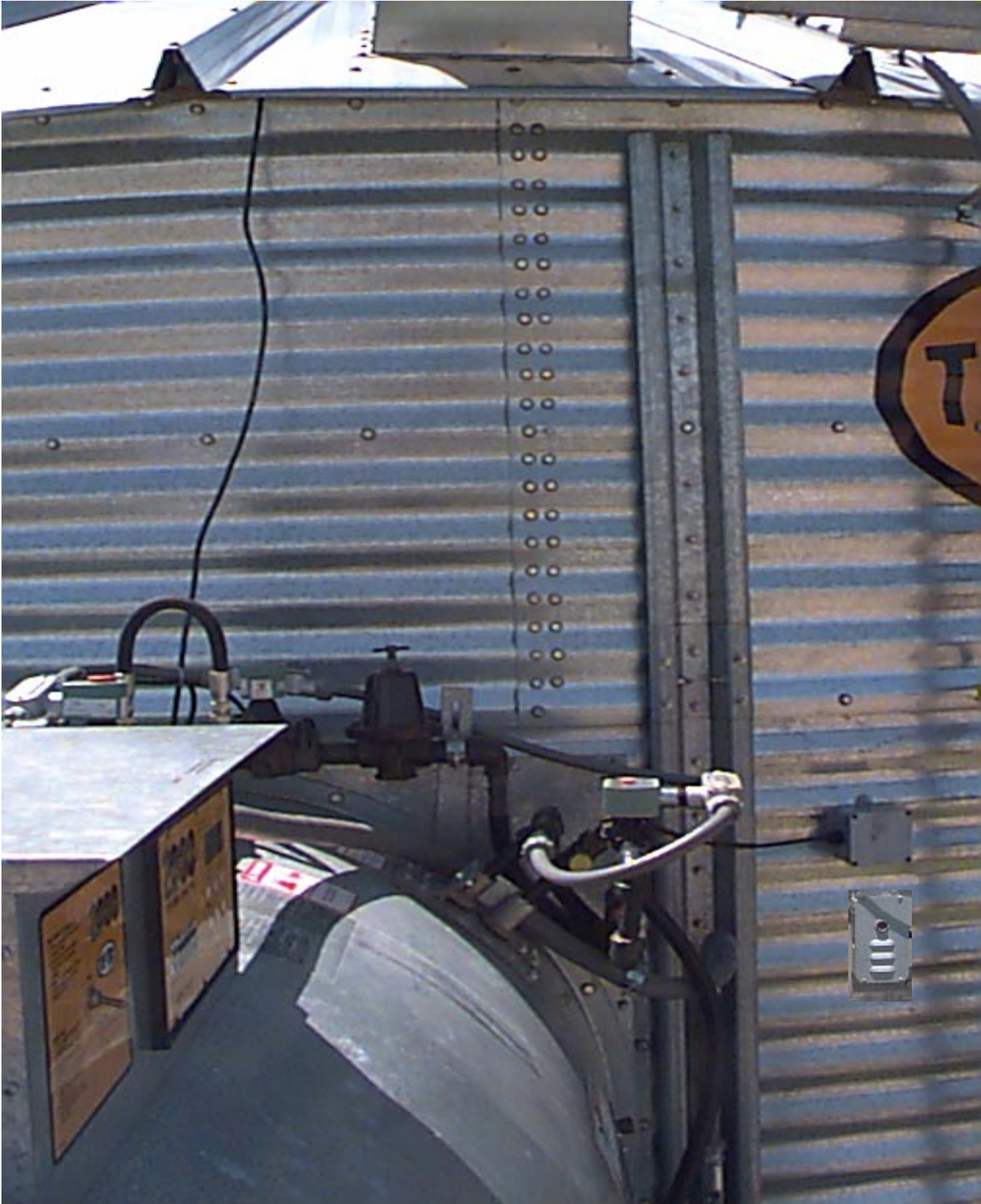
Fan/heater unit mounted to the bin, showing the plenum high limit, the airswitch, and cord going through the eave to the grain temperature sensor brackets.
